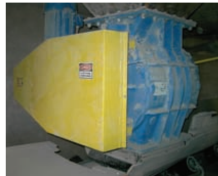
The chain and sprocket that drive the valve's rotor are protected by an OSHA-yellow cover.
