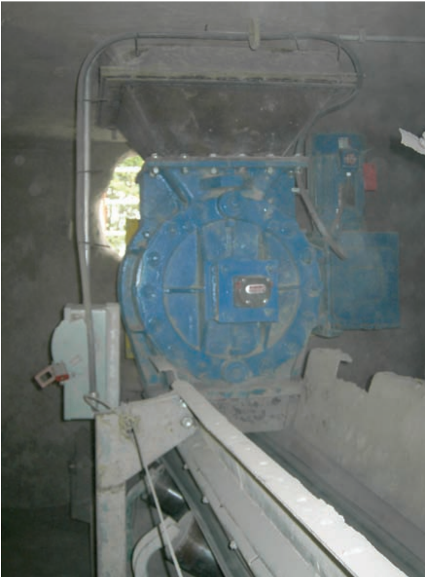
The new severe-duty rotary valves feed the gypsum from a storage silo to a belt conveyor.
